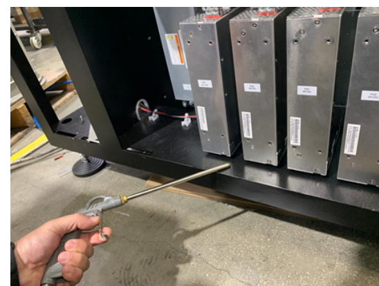
Figure 10-2 Clean Power Supply
