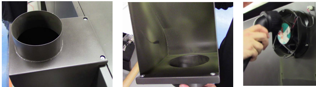
Figure 9-4 Metal Exhaust Vent Housing (Left and Middle) and Vacuuming Exhaust Fan (Right)
