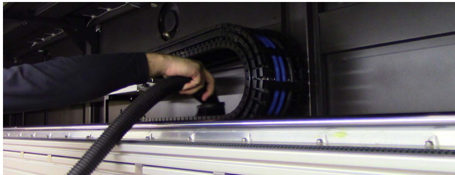
Figure 9-3 Vacuuming Cable Carrier
